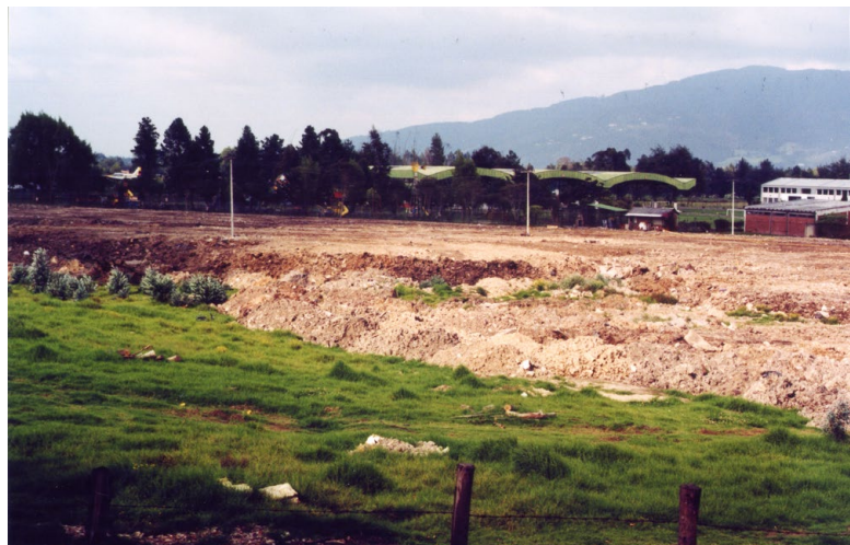
Figure 4.6. Process of filling the floodplain of Tibabuyes between humedal La Conejera and Juan Amarillo River with rubble and construction debris for urbanization.
