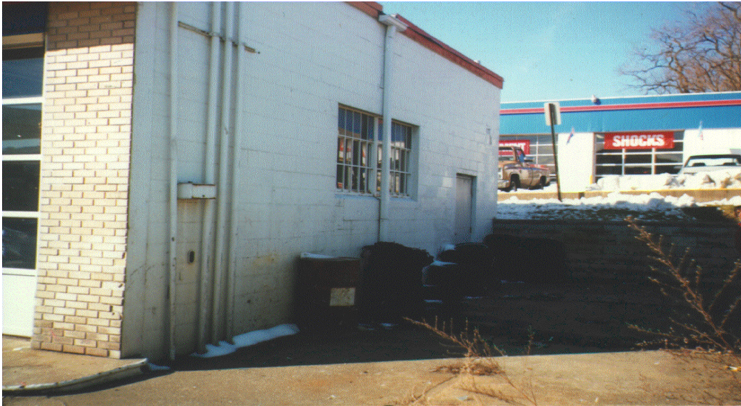
Figure 5.2: Photo showing 55-gallon drum and used tires on side of building
